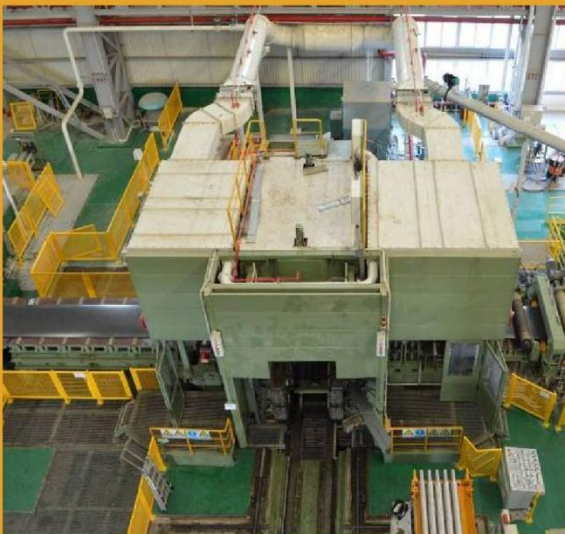
In line mill 2E在线轧机 Sungwig /Andritz (Austria) Reduction(压下率):30%
