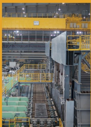
Reheating Furnace 加热炉 CISDI(China) Thickness(厚度): 200mm&220mm
