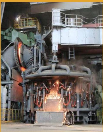
EAF 电弧炉 SMS-Siemag (Germany) 160MT per charge 吨/炉
