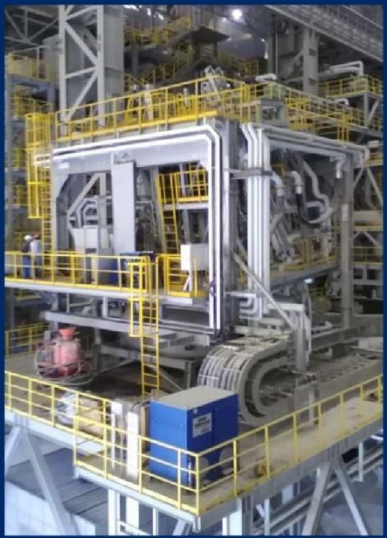
VOD 真空精炼炉 SMS-Siemag (Germany) 180MT per charge 吨/炉
